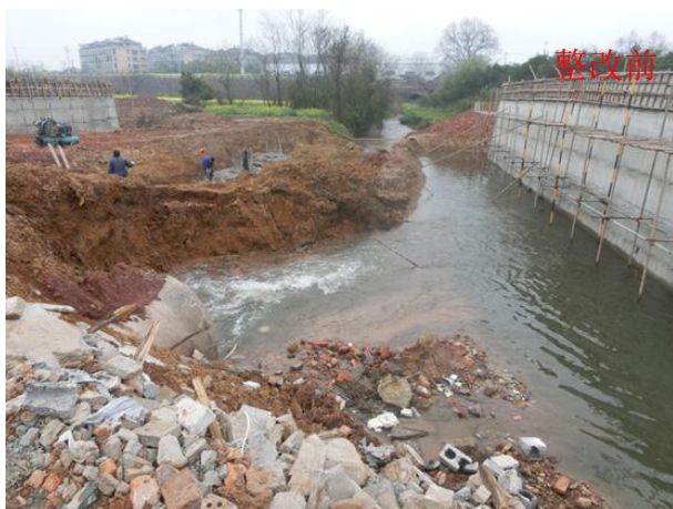
图 1-76 寺落潭桥边坡被河水冲刷 (2018.6)
