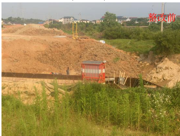
图 1-78 K20+700 处边坡裸露 (2018.6)
